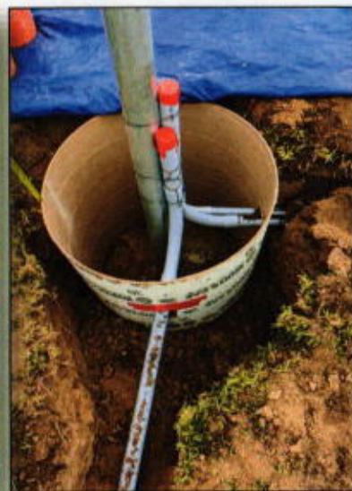
Conduit Run From 1 st Field Radar to 2 nd Field Radar
