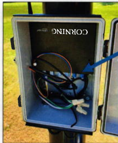
Example Showing the Inside of the Fiber Junction Box with Fiber Patch Panel
