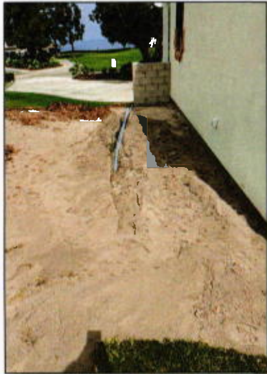
Conduit to Server Rack Building
