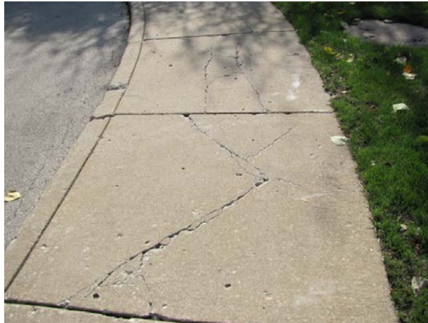
Concrete sidewalk cracks
