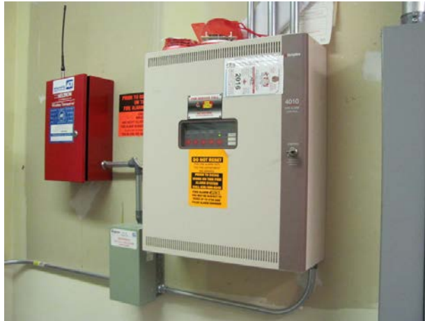
Life safety system control panel
