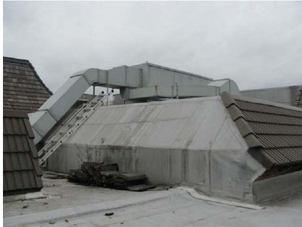
Make-up air unit
