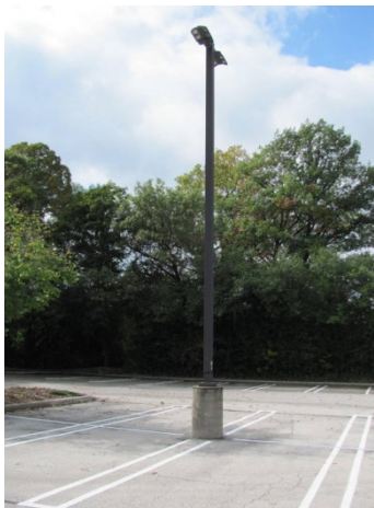
Light pole and fixtures at parking area
