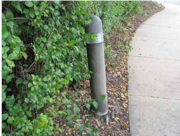
Lean and finish deterioration
