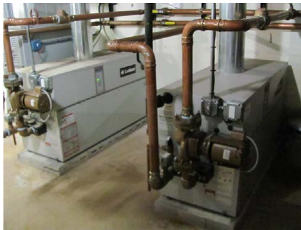
Domestic hot water boilers
