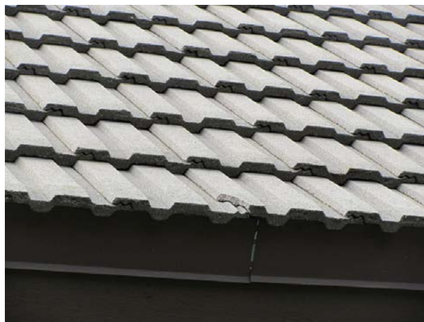
Isolated cracked tile at addition
