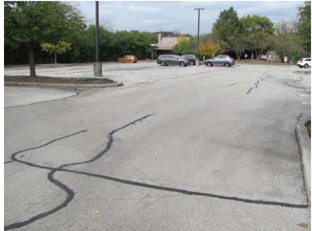
Asphalt pavement parking area, note crack repairs
