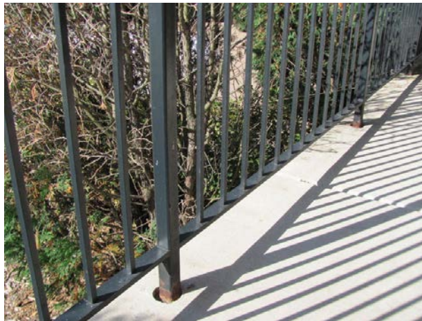
Rust at steel railing post, note - post pockets should be sealed to shed water away from post
