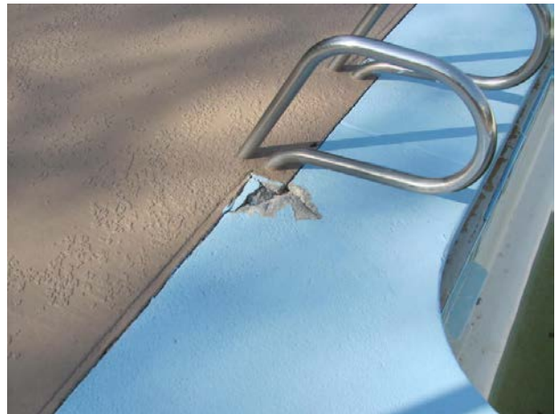
Spalled concrete coping
