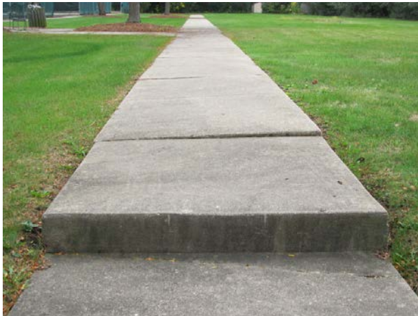
Concrete sidewalk settlement
