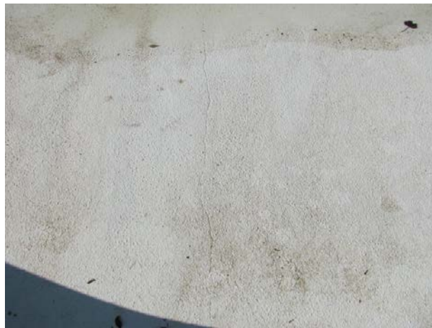
Plaster crack and stains at wading pool
