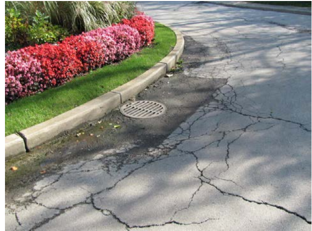
Significant deterioration surrounding catch basin
