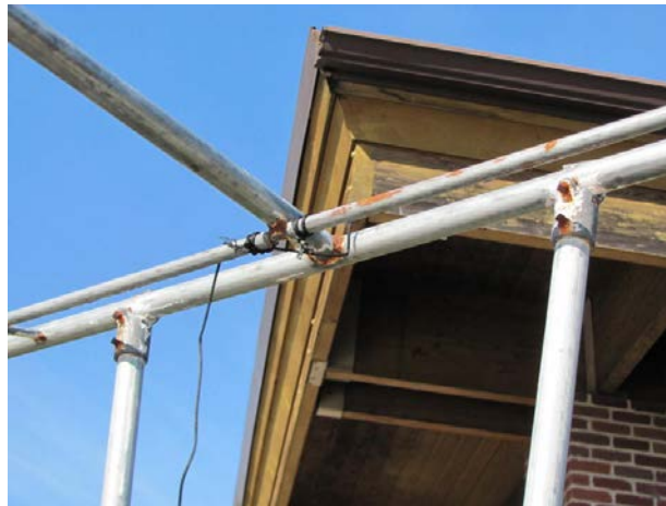
Typical rust at frame
