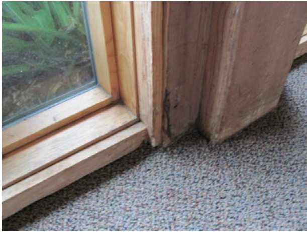
Typical water stains at dining room interior
