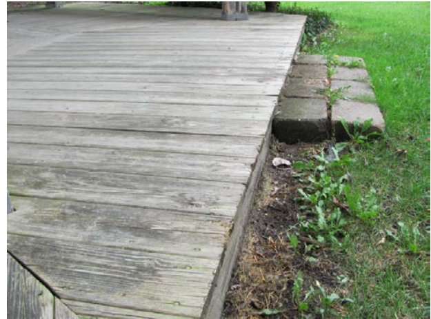
Weathered deck boards
