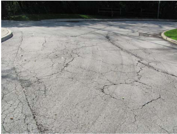
Typical cracks and raveling at circle access drive
