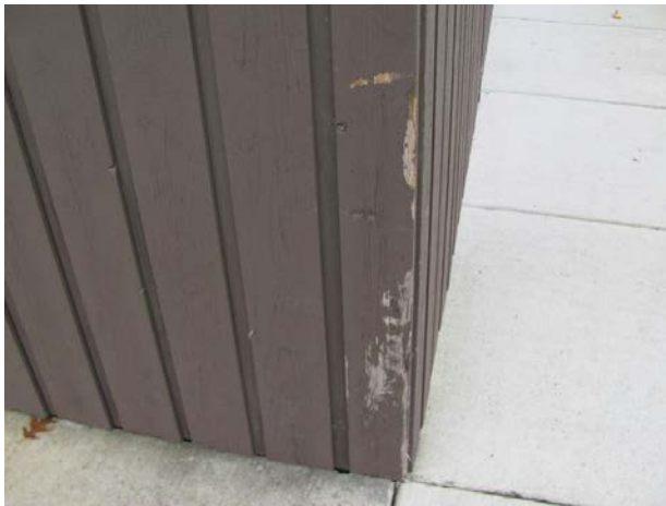
Damage at addition
