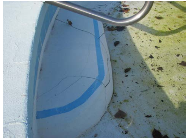
Multiple cracks at wading pool step
