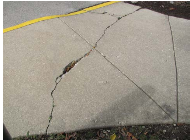
Concrete sidewalk cracks
