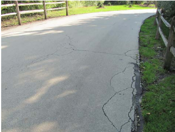
Asphalt pavement access drive, note edge deterioration
