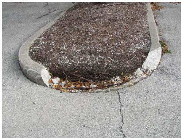
Damaged concrete curb
