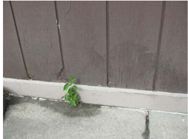
Typical wood rot at siding, note - accelerated deterioration at bottom likely caused by contact with storm water runoff from south
