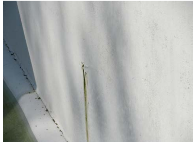
Possible location of seepage at diving pool
