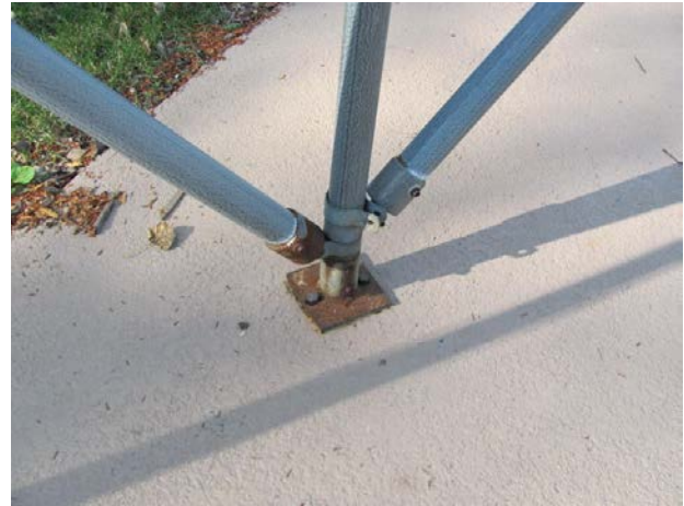
Typical rust at post fastener
