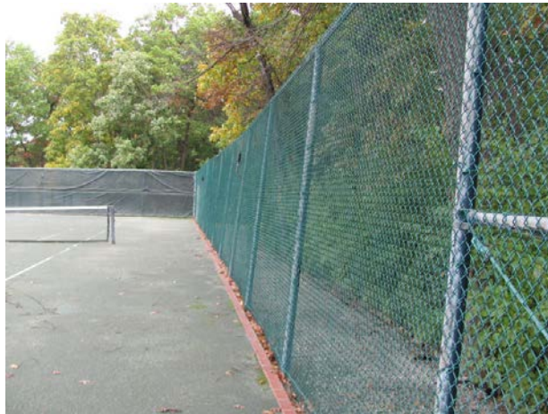
Leaning fence at courts 6-8
