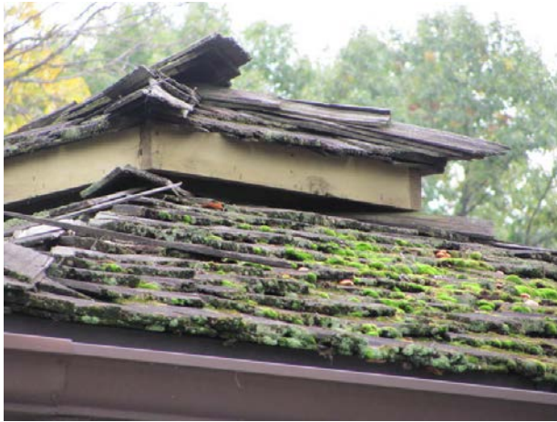
Cedar roof mildew growth and deterioration
