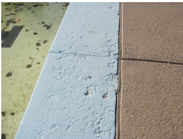
Spalled concrete coping
