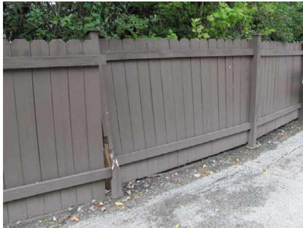
Damaged wood fence
