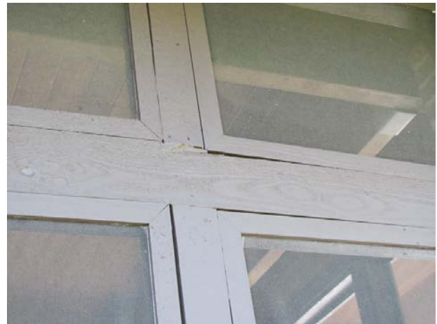
Damage at screened-in porch
