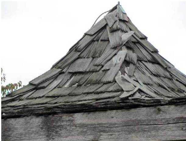
Cedar roof deterioration
