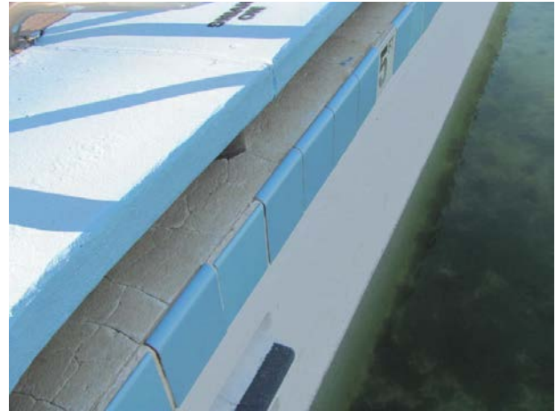
Replaced and mismatched tiles
