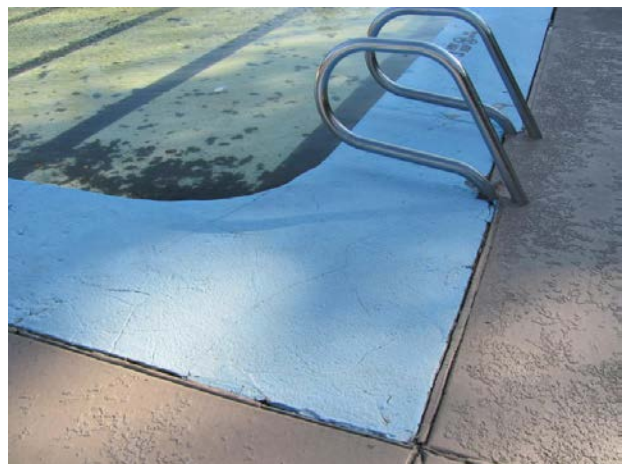
Multiple cracks at coping
