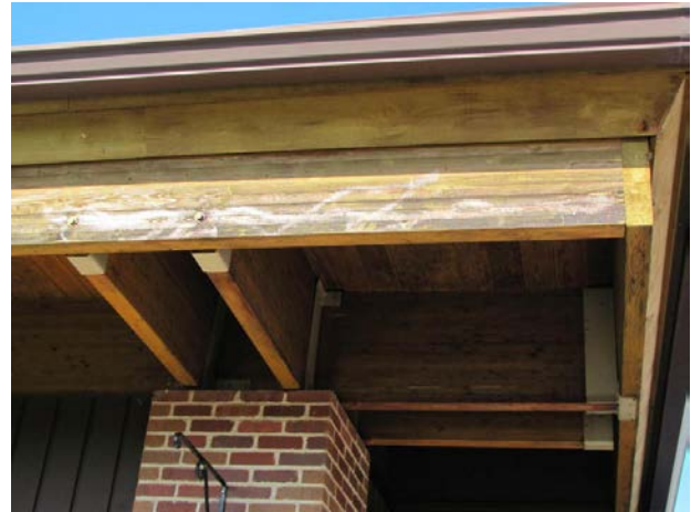
Faded and worn stain application
