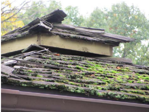
Cedar roof mildew growth and deterioration
