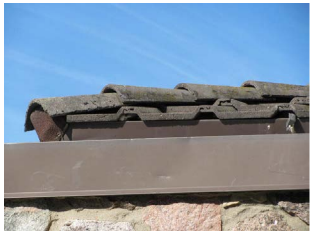
Spall evident at older concrete tiles
