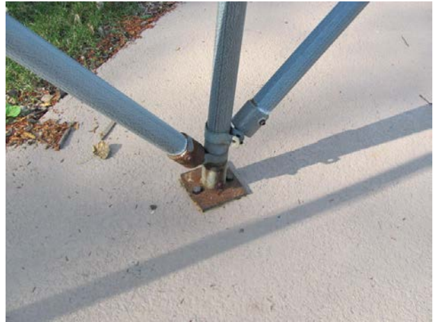
Typical rust at post fastener
