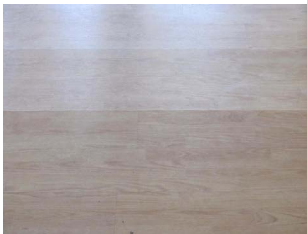
Warped wood laminate floor covering
