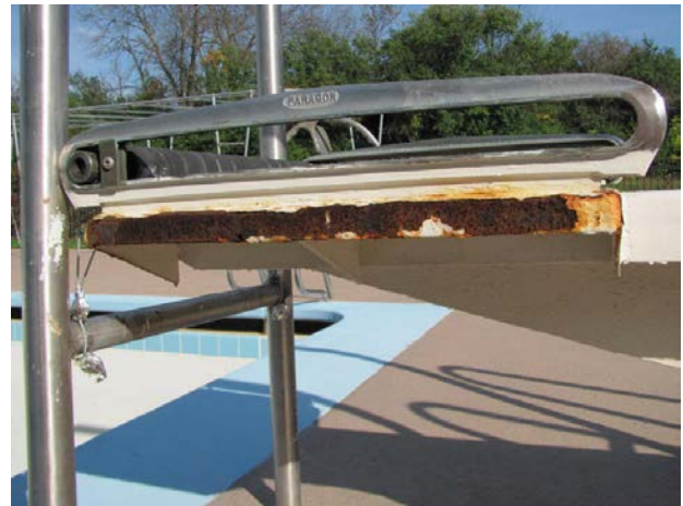
Corrosion evident at diving stand
