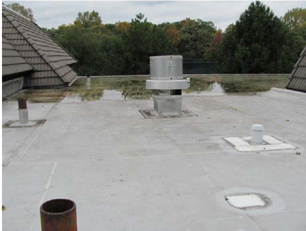
Standing water at EPDM roof
