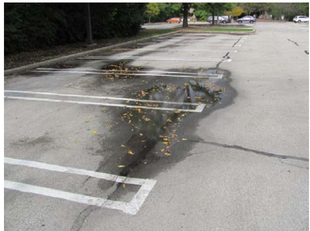
Standing water at settled pavement
