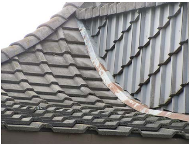
Older concrete tiles, note rust at flashing
