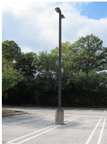
Light pole and fixtures at parking area
