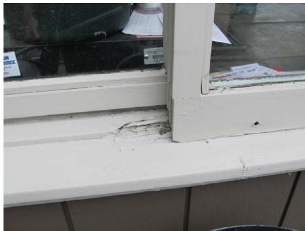
Wood rot at window
