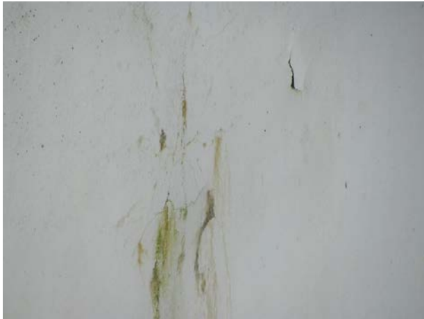
Possible location of seepage at diving pool
