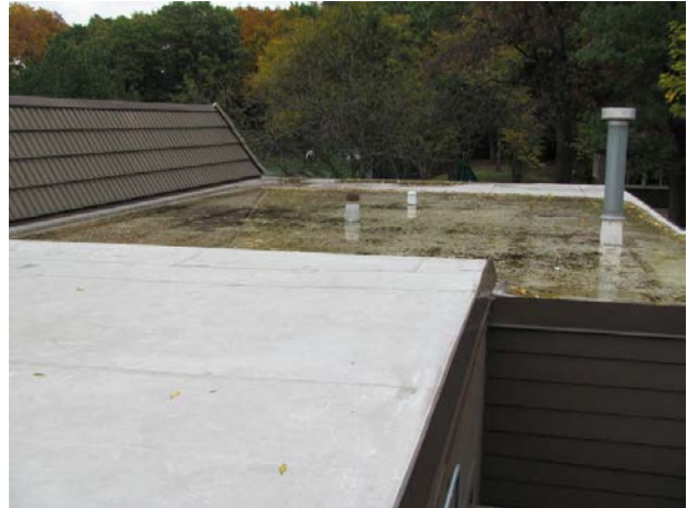
Standing water at EPDM roof
