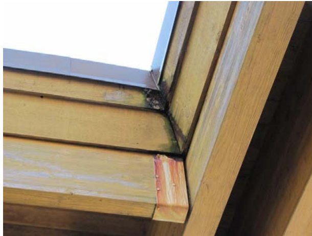
Accelerated wood deterioration caused by roof drainage at porte-cochere
