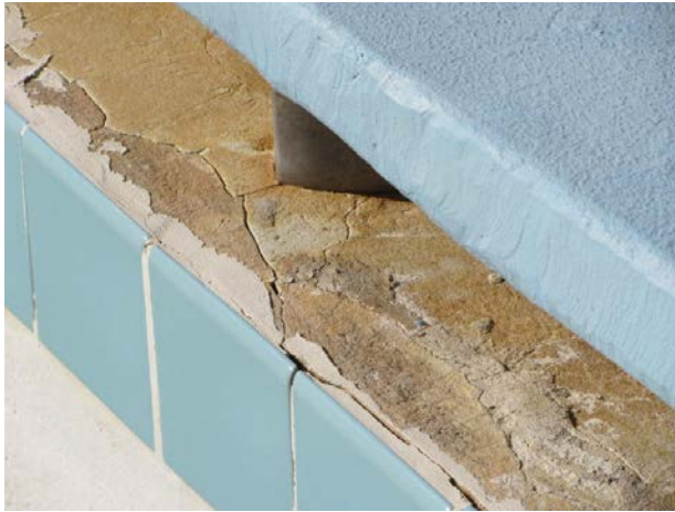
Typical concrete cracks at gutter system
