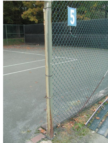
Rusted fence post at court 5
