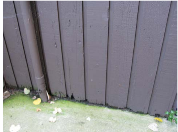
Wood rot at original building
