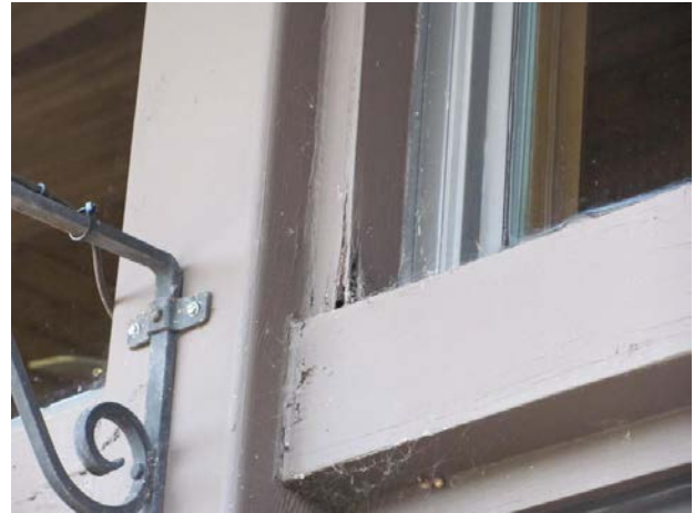
Wood rot at column
