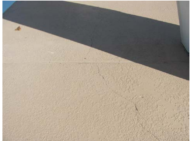
Concrete cracks near diving stands
