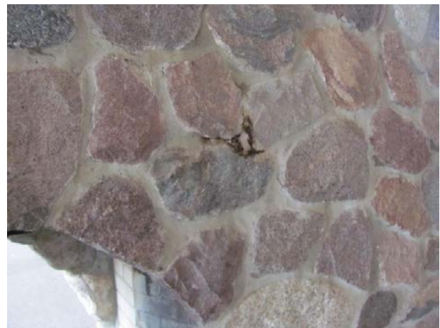
Seepage at interior
