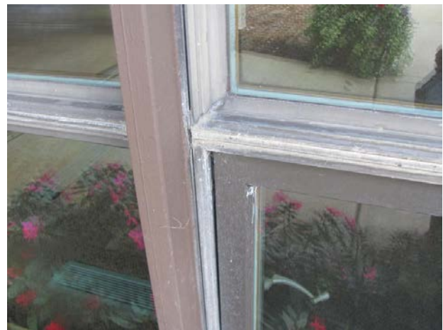
Frame finish deterioration
