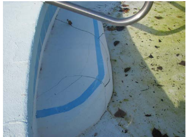
Multiple cracks at wading pool step
